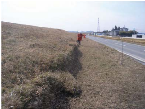
Figure 4. Naruse River, R12.0k (River division, NILM). The levee spread laterally on the surface of foundation soil toward hinterland side. There was not any detected deformation outside the levee toe.
