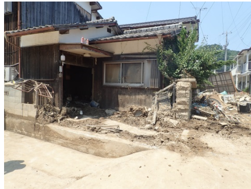
写真⑪(家屋崩壊)
